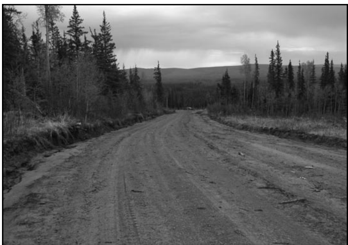
Same segment of road after breakup. (Photo by Steve Joslin)
