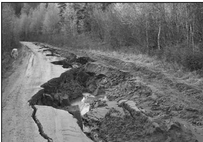
Eroded road prior to chip treatment. (Photo by Steve Joslin)
