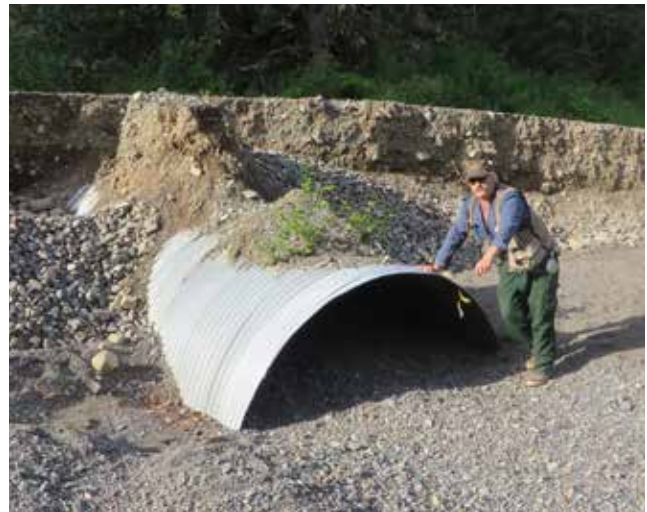
John Winters, Forester II, Kenai-Kodiak Area on FRPA Inspection. This culvert doesn't work!
