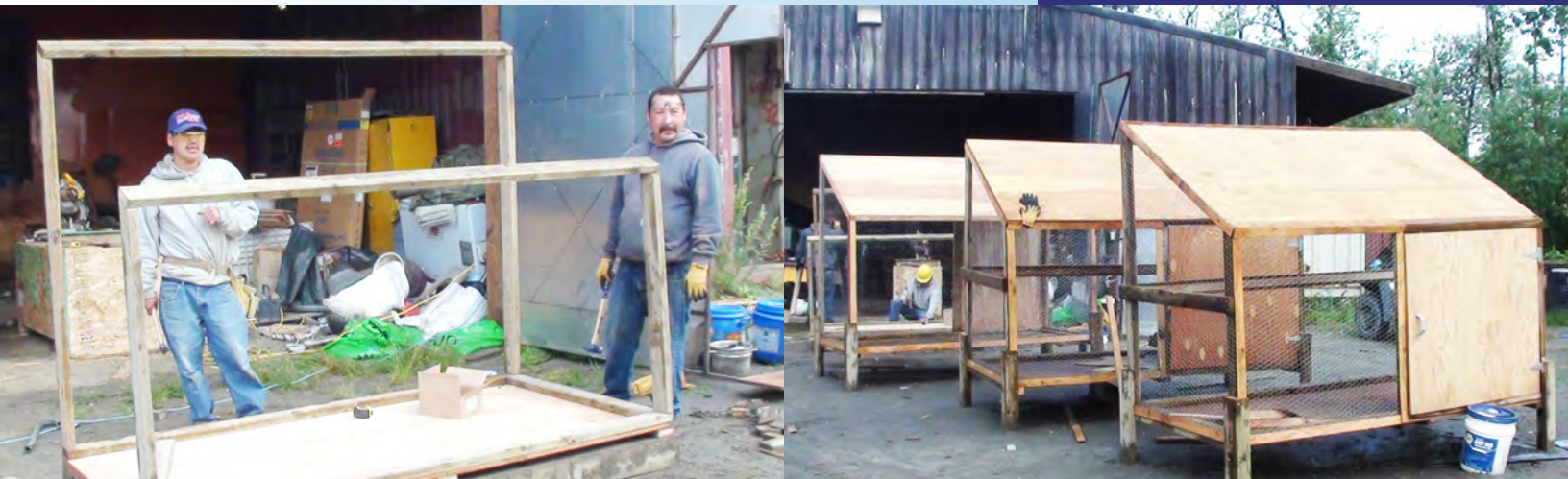
Enclosed collection bins are built off the ground to keep waste contained and animals out of the trash. Photos by Lena Foss
