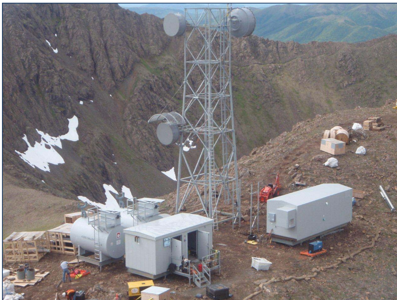
Caribou Ridge Microwave Repeater - Enhancing telecommunications in rural Alaska.
