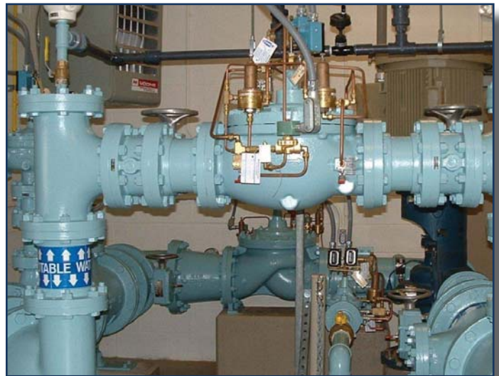
Interior piping at AWWU’s Service High ten million gallon reservoir.
