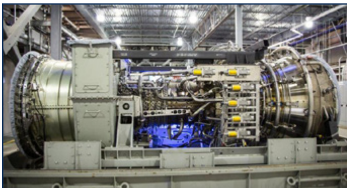
A LM6000 Turbine at SPP
