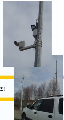
DOT# READERS ON NEW SEWARD HIGHWAY
