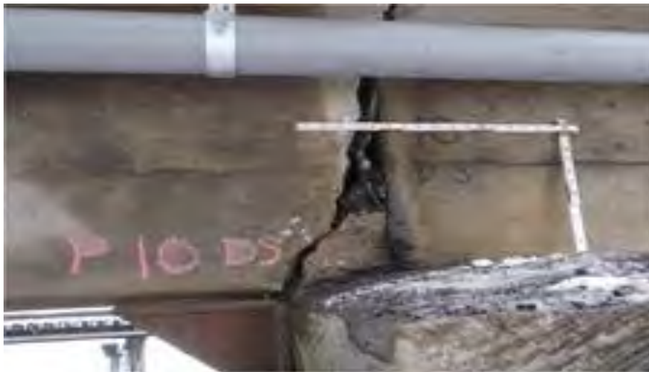
Figure 6. Deteriorating Concrete Trail River Bridge
