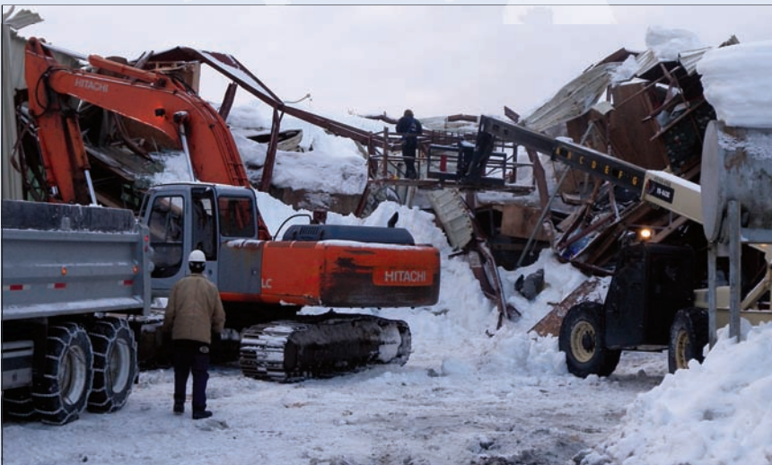
Roof Collapse. A crew works to salvage what they can from an unoccupied building in Cordova after the roof collapsed. Damages to homes, private boats, city buildings and facilities, the Cordova Medical Center, commercial buildings, schools and infrastructure were reported by the city of Cordova. Photo: Karl Edwards, DHS&EM
