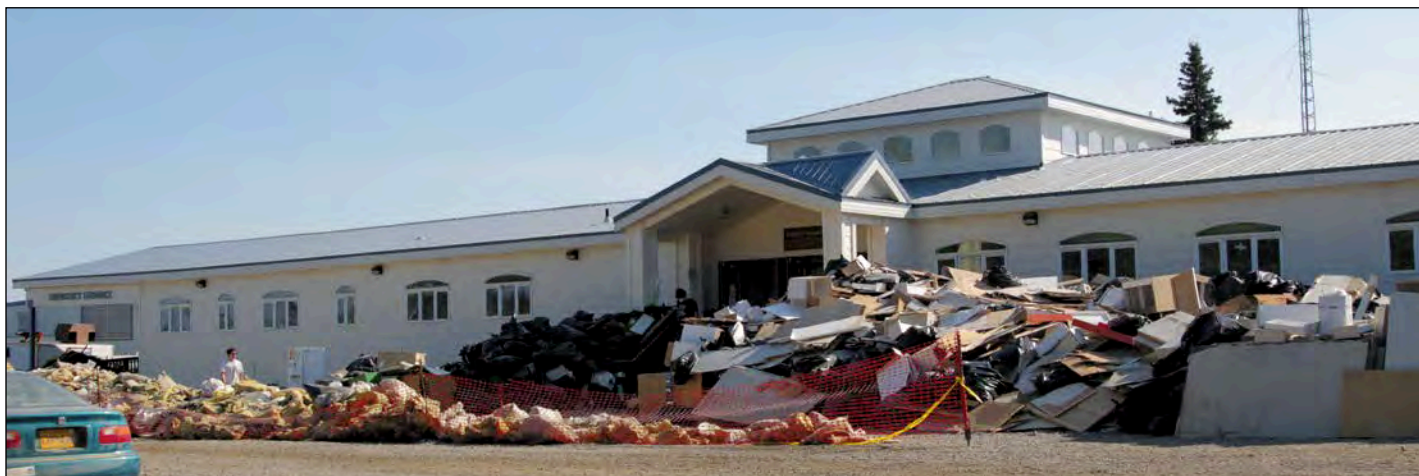
Debris Removal. Insulation and debris mount outside the Galena city hall building and health clinic in June, as workers cleared out the building down to the studs because of the damage caused by flooding. Photo: Kalei Rupp, DMVA Public Affairs
