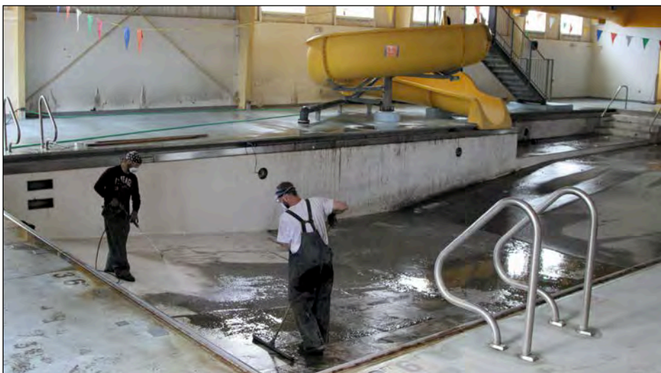
Pool Clean Up. Workers clean up the community pool in Galena in June after flood waters from the Yukon River damaged the facility as well as many homes and other public buildings in town. Photo: Jeremy Zidek, DHS&EM
