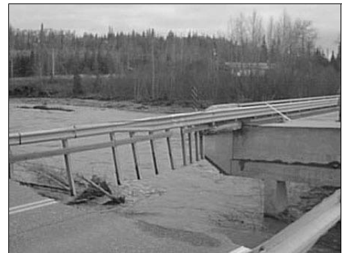
Alaska disasters in 2002 included October flooding on the Kenai Peninsula, where roads were washed out in Ninilchik (top) and in the Deep Creek area.
