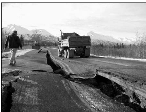
Above and right: Damage to the Tok Cutoff from the Nov. 3, 2002, earthquake.
